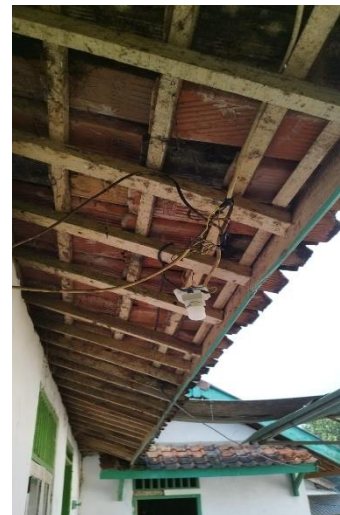
c. Kondisi outdoor
